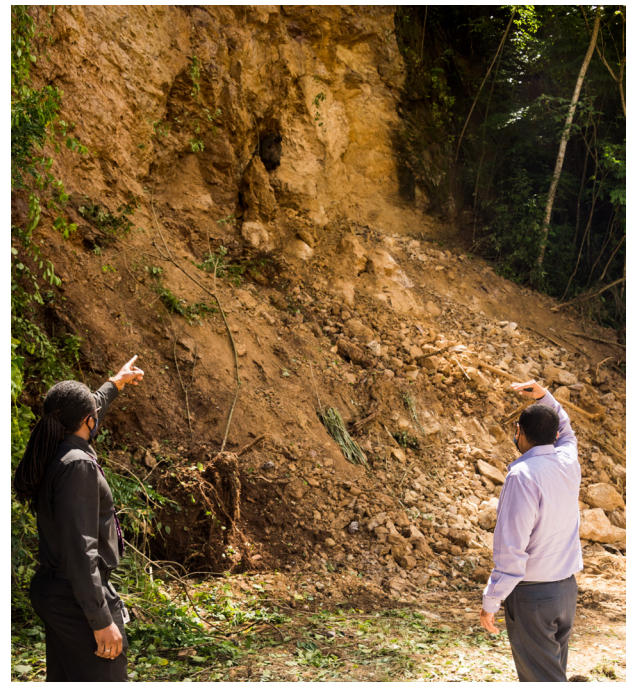
Senator the Honourable Rohan Sinanan Minister of Works and Transport (right) and Jimelle Wilson (left), St. George West District Engineer of the Highways Division examine the aftermath of the landslide at the North Coast Road.
