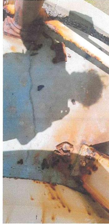
Pic. 13 Crack in the cantilever slab
