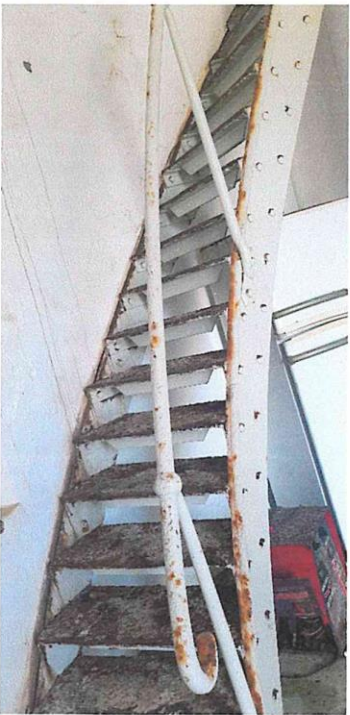
Pic. 14 Corrosion of ground floor ladder
