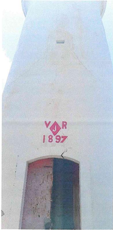
Pic. 20 Western face of lighthouse showing vertical crack
