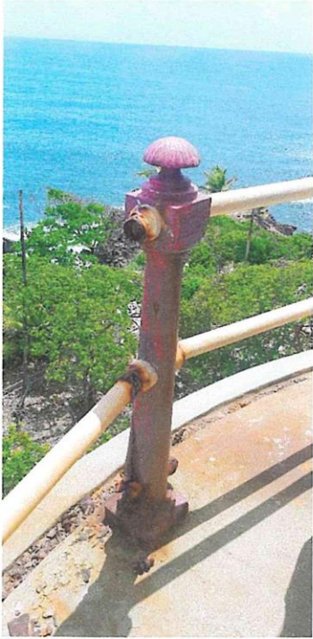
Pic. 12 Corrosion of the metal hand rails of the cantilever
