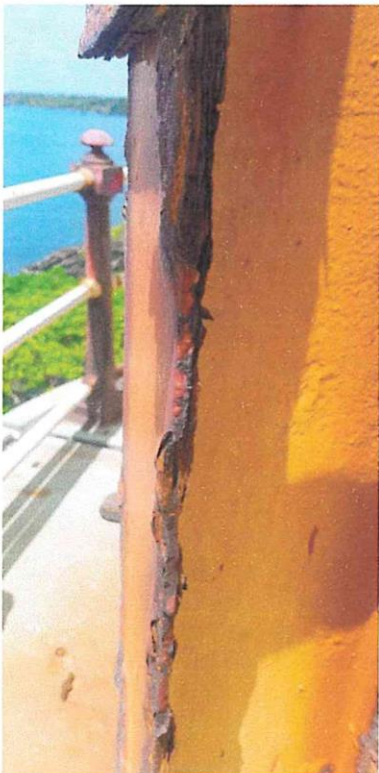
Pic. 10 Cantilever slab and corrosion of steel member
