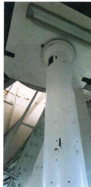
Pic. 4a. Top of vertical pipe connected to the soffit of the 3 rd floor
