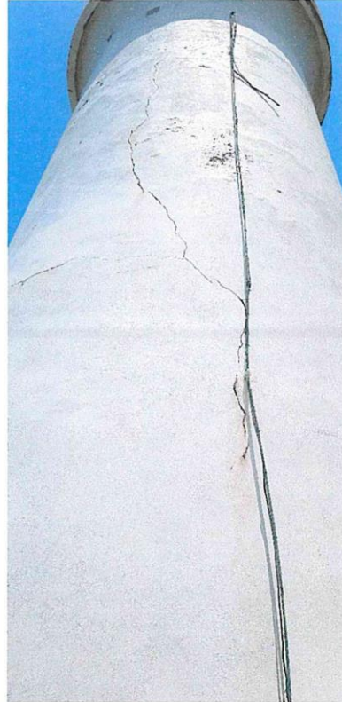
Pic. 17 Cracks of the external protective paint at the eastern face of the lighthouse
