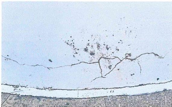
Pic. 18 Cracks of the external protective paint at the base of the eastern face of the lighthouse
