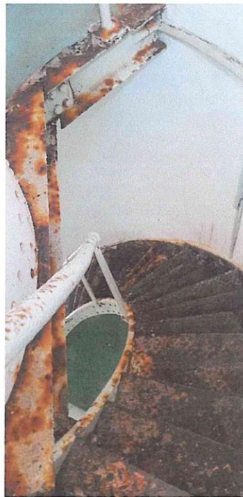
Pic. 15 Corrosion of first floor ladder
