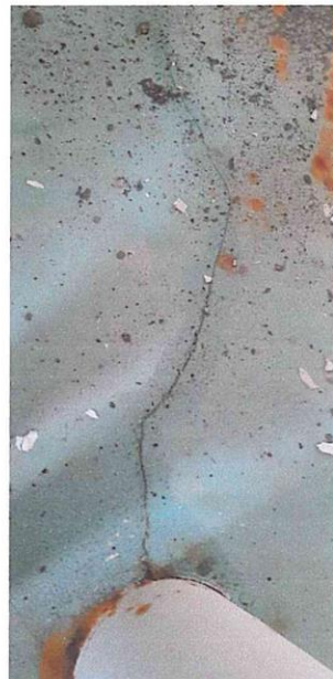
Pic. 19 Typical crack on the suspended floor slabs
