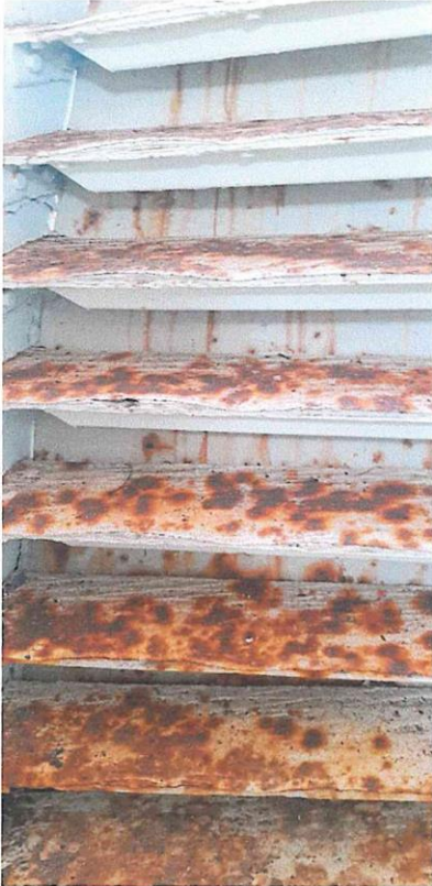
Pic. 16 Corrosion of second floor ladder
