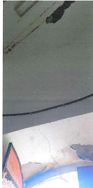
Pic. 21 Crack at soffit of doorway lintel
